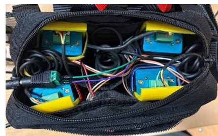
Figure 7 – Wiring and cable management system
